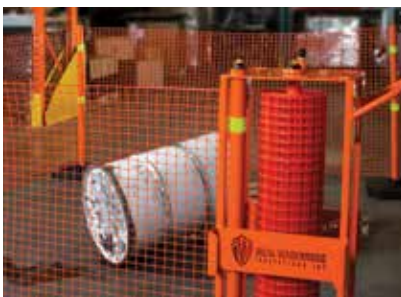
SECURE A TEMPORARY HAZARDOUS AREA
