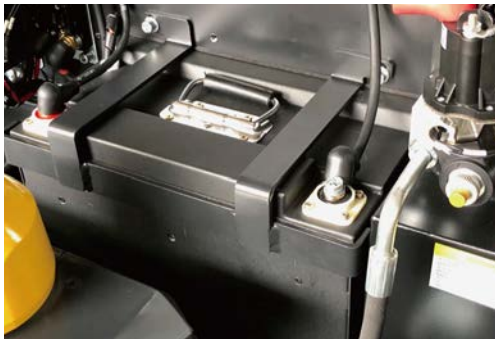
24V/60Ah Lithium-iron battery has connection terminals with screws and is protected inside the steel case.
